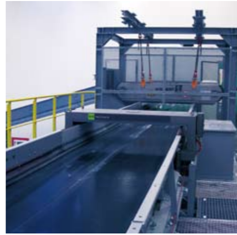
Flat belt conveyor with peripheral equipment
