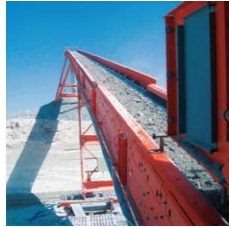
Throughed belt conveyor
