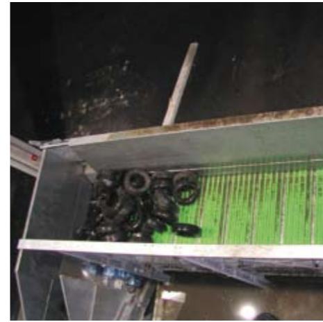
Feeding bunker slat conveyor
