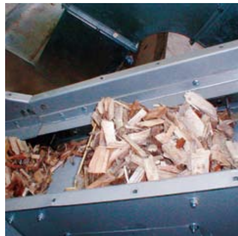
Troughed chain conveyors
