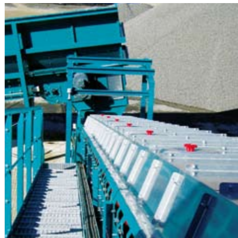
Cavity belt conveyor with inspection and hood covering
