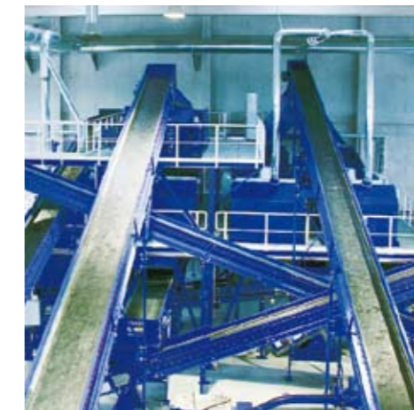
Complete conveyor systems
